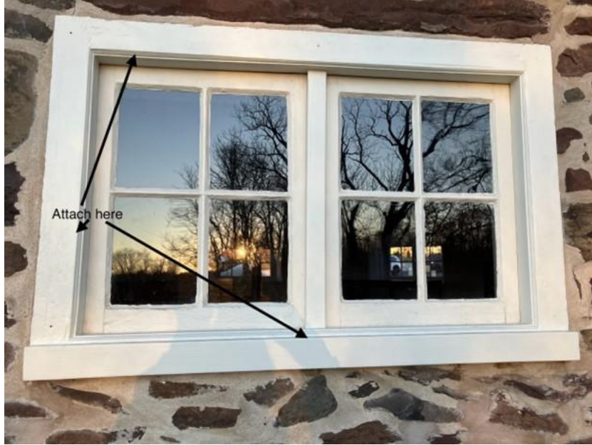
Proposed placement and attachment locations for installing metal frame storm windows on existing window frames of Octagonal School (photo diagram by Jane DelBianco).
