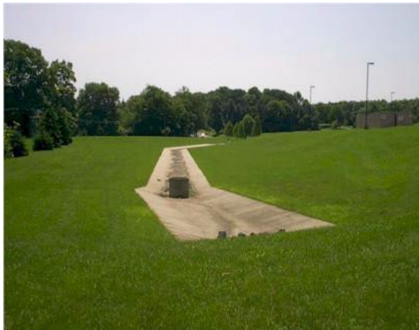
Figure 9-25. Existing sinkhole-plagued detention basin.
