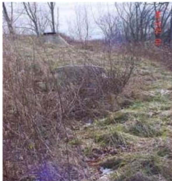
Figure 9-35. This trench/berm has a subsurface energy dissipater to reduce the velocity of entering stormwater.
